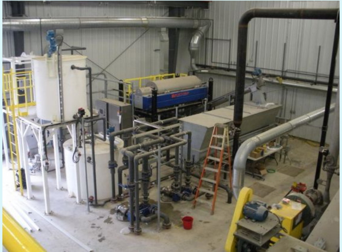
Liquids/solids separation facility
